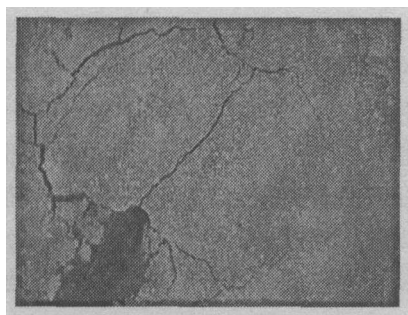
图 6 外径为 76 mm 桩形成的鼓包 Fig.6 The bulging formed by a 76 mm diameter pile
